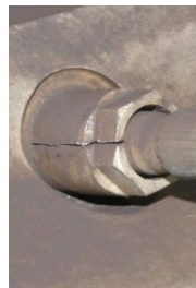
Sensor with cracked nut
